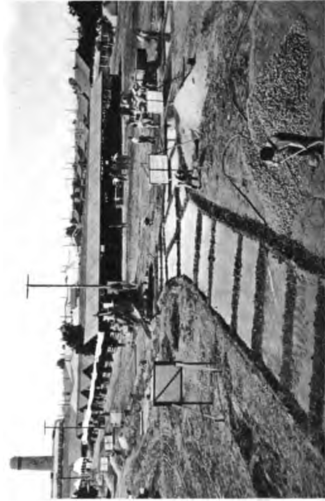
Demonstration concrete highway put down during State Fair at Sacramento. This educational work was carried on during the 1916 State Fair by the California Highway Commission co-operating with the Sacramento County Good Roads Association to boost the County bond issue.
